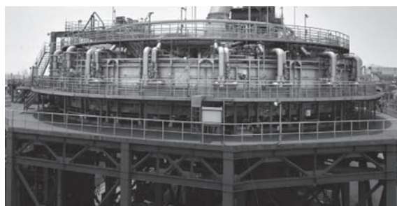
Fig.8 FASTMET Commercial Plant at JFE Nishinohon Works
