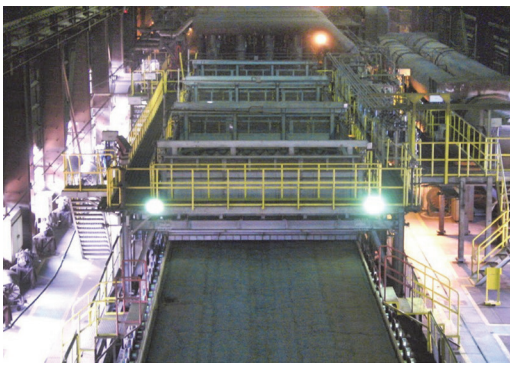
Fig.3 Equipment of gaseous fuel injection technology in Keihin No.1 sinter plant.
